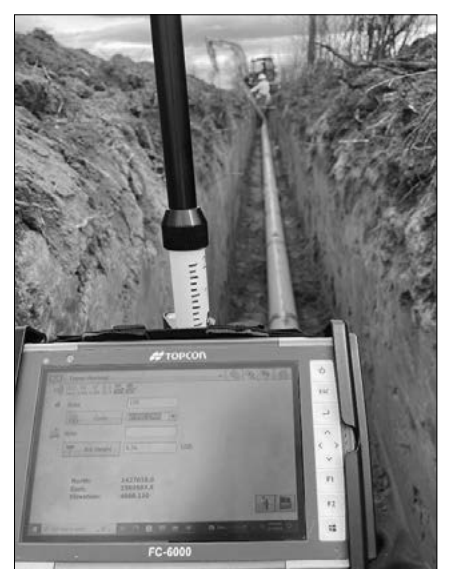
GPSing of new water line installed to add to the Utility Map
