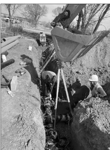
Gate Valve installation to isolate main water line in case of emergency
